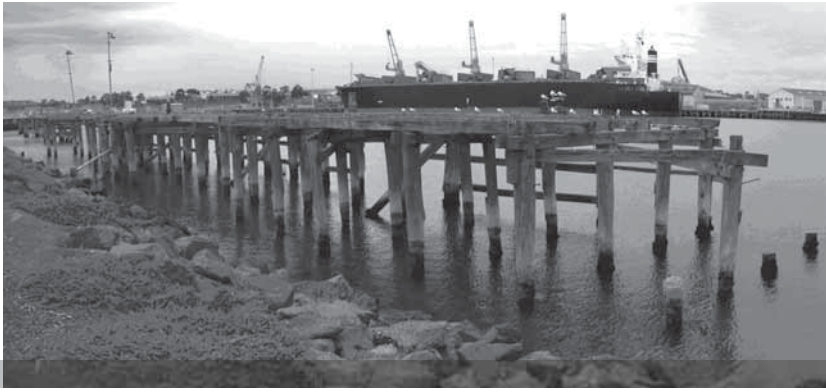
Remains of the Corio Freezing Works and Abattoir Wharf (H7721-0147) in 2004. Heritage Victoria.
